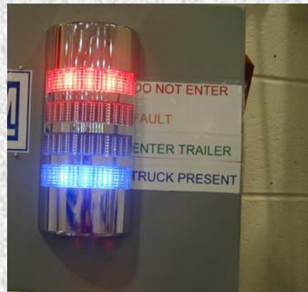
Dock Communication Systems
